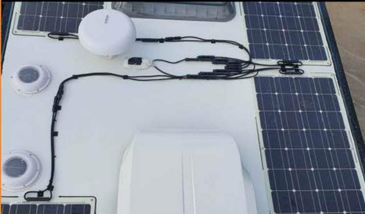
4 x 100W roof mounted solar panels.
